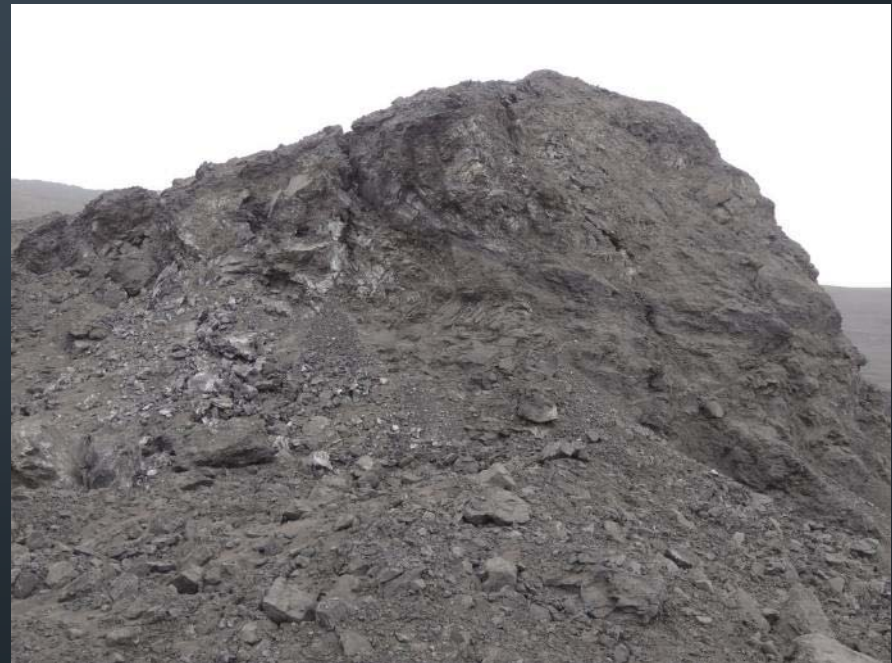
Sheared and faulted zone along part of the eastern flank of failure
