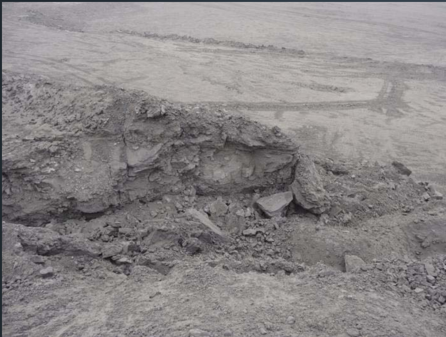
Near bottom corner of failure
